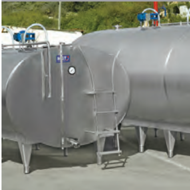
Cooling & storage tank
