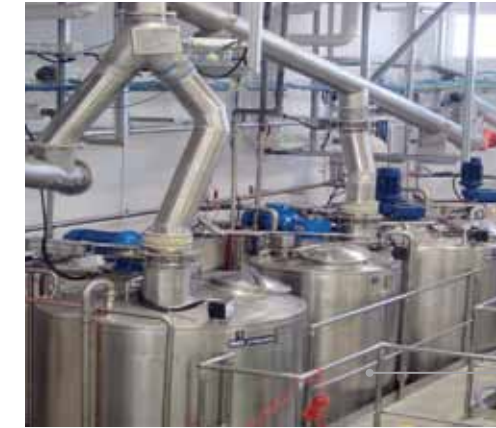
Tanks working platform and sugar conveyor
